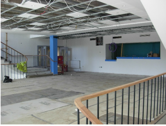
First floor bar and circulation area – original parquet flooring is being retained and refurbished
